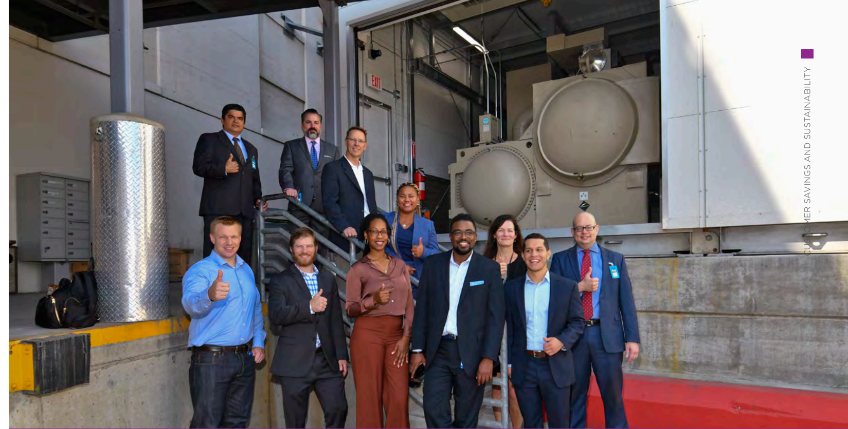
CoreSite's downtown Los Angeles facility, LA2, earned 1 st Place in the Energy Efficiency Excellence Award category at LADWP's 2020 Sustainability Awards, along with a $3 million rebate check from LADWP helping to defray the cost of the efficiency measures. CoreSite conducted an extensive cooling retrofit that replaced its chilled water-cooling system with a new, centralized water chiller system consisting of four 1,500-ton water cooled chillers. The project also included installation of variable speed cooling towers, variable speed chilled water and condenser water pumps and water-side chiller heat exchangers. The efficiency upgrades are expected to save nearly 10 GWh annually.
